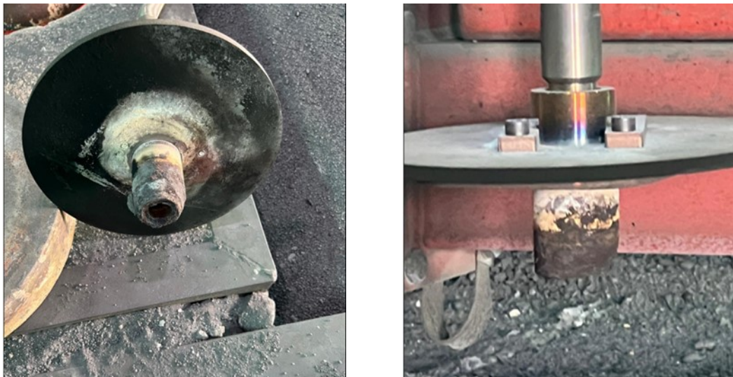
Figure 8. Burner nozzle condition after 9 months of Service.
